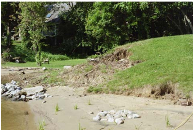
Figure . Epping Forest, Section 1, bank erosion
